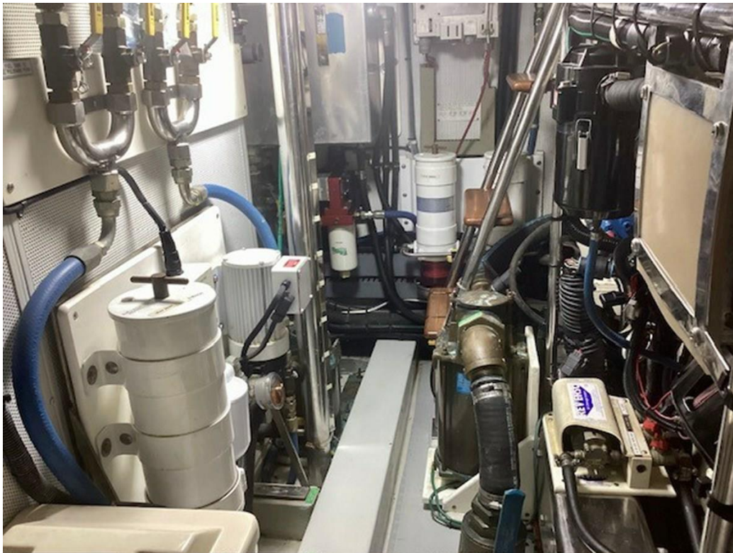
2005 Selene 53 (ASANTE) Engine Room
